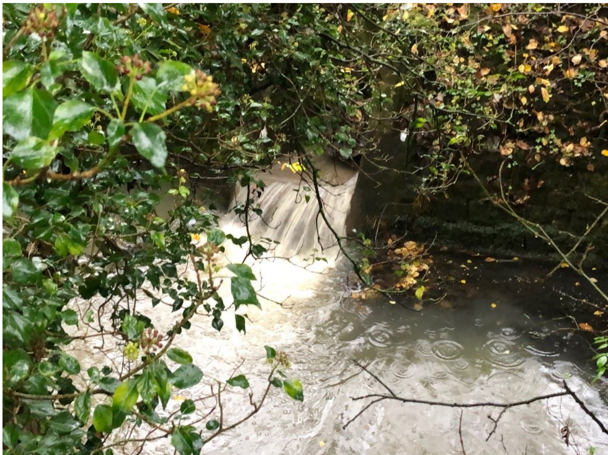
Figure 5. Untreated effluent overflow from Addingham Pumping Station on 29 th October 2010
